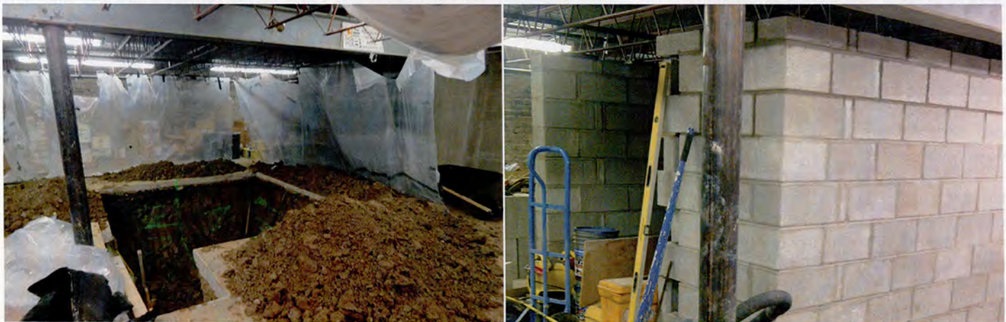
The elevator has progressed from a hand-dug hole in the basement and is now ready to reach up through the first and second floors.
